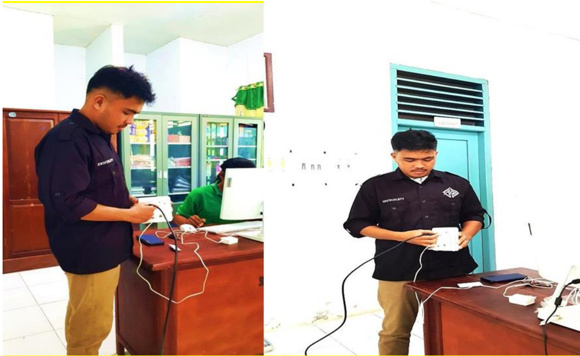
Gambar 5. Coaxial Cable Installation Process - Antenna - Modem
